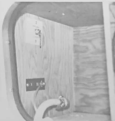
Cable TV Terminals
